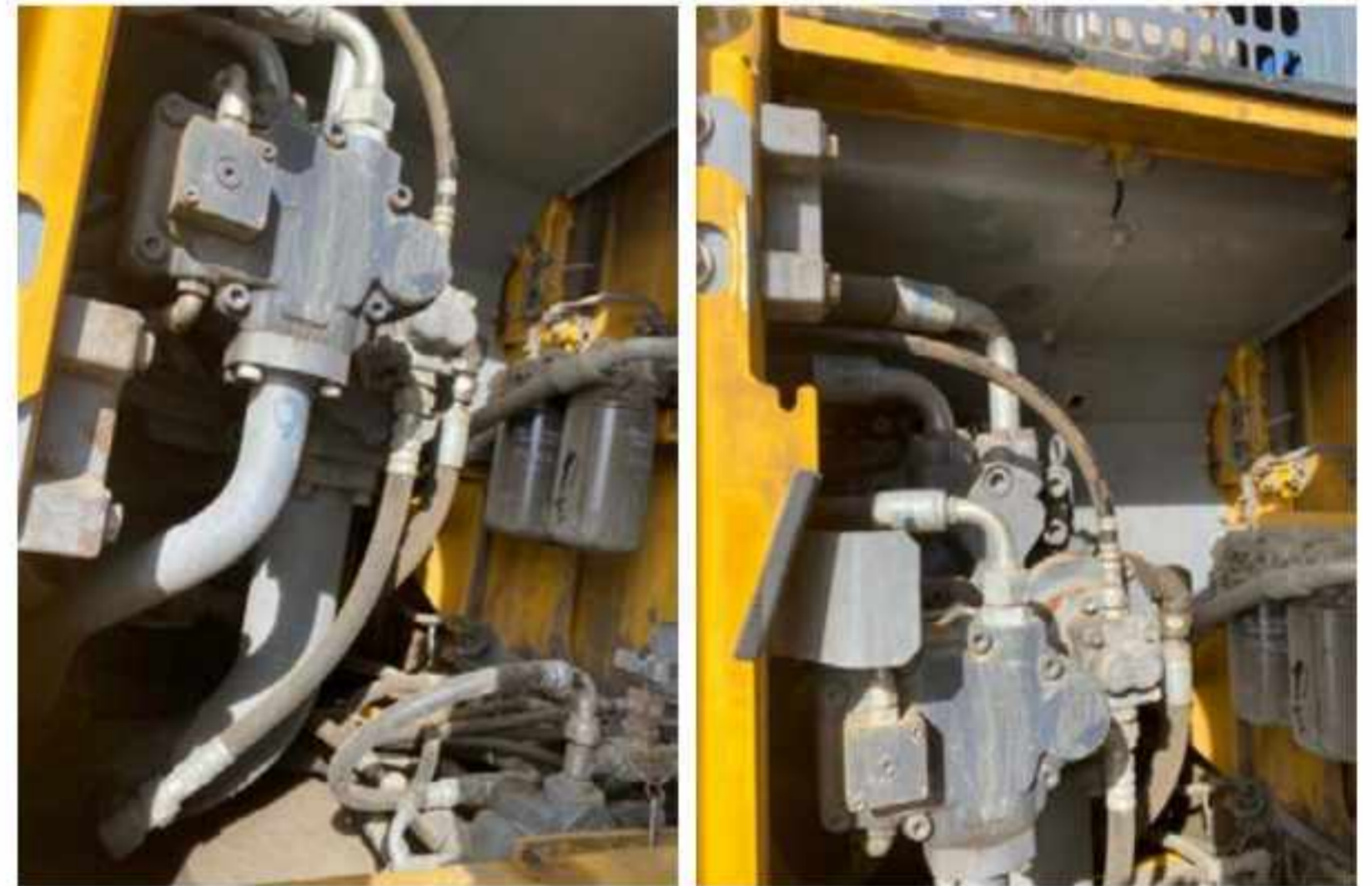
Hydraulic Leaks Photos
